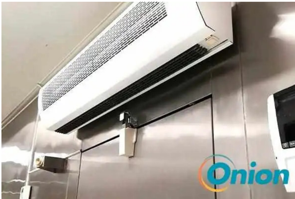
Weyland kitchen cooling solutions klimaanlage
