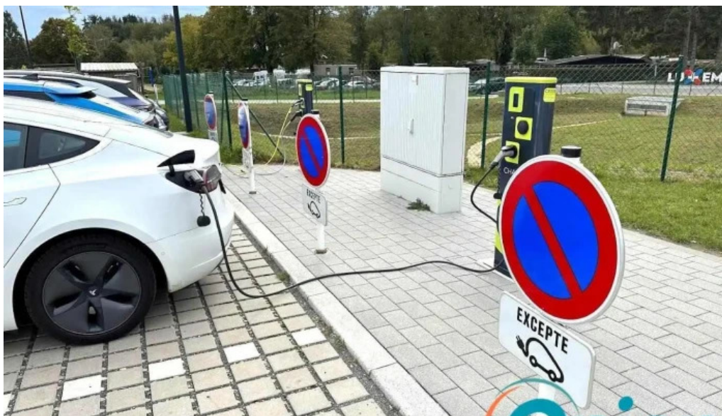
Chargy ladestation berdorf
