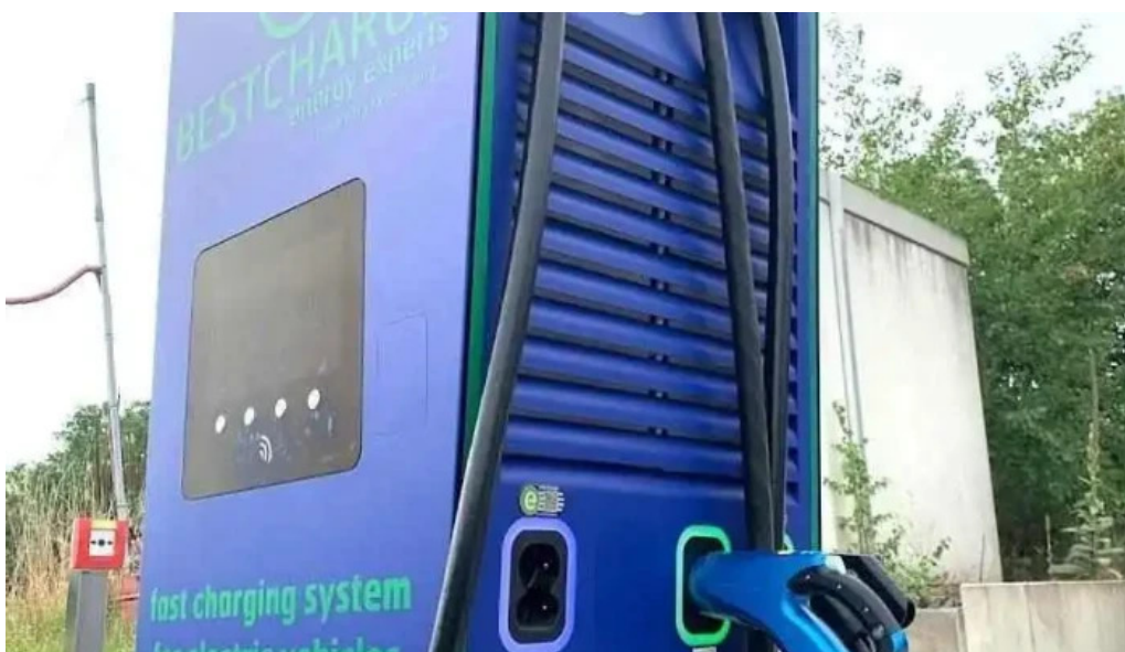
Bestcharge charging station esch sauer
