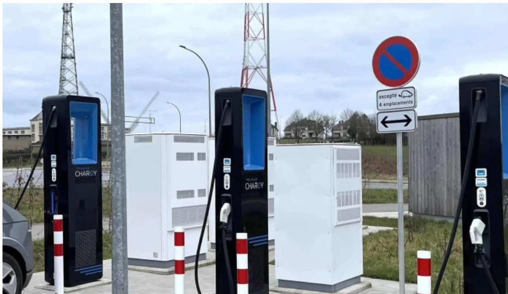
Charge charging station kommentaren
