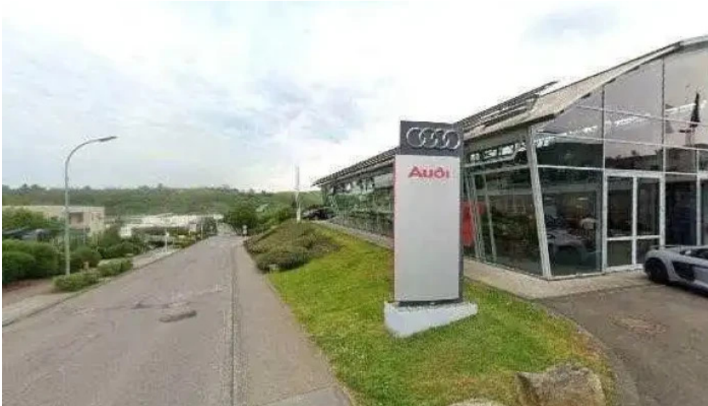
Losch import sarl charging station nummere
