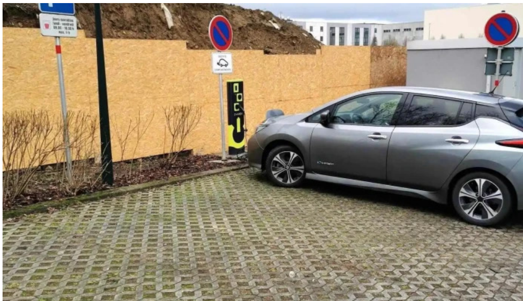
Chargy charging station praisserie
