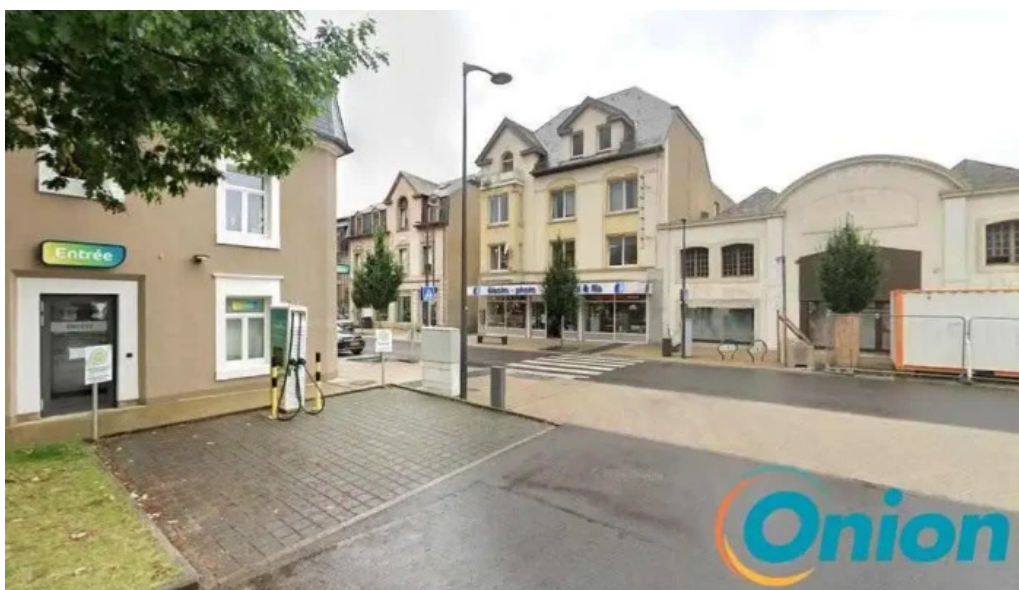
Creos luxemburg charging station mersch
