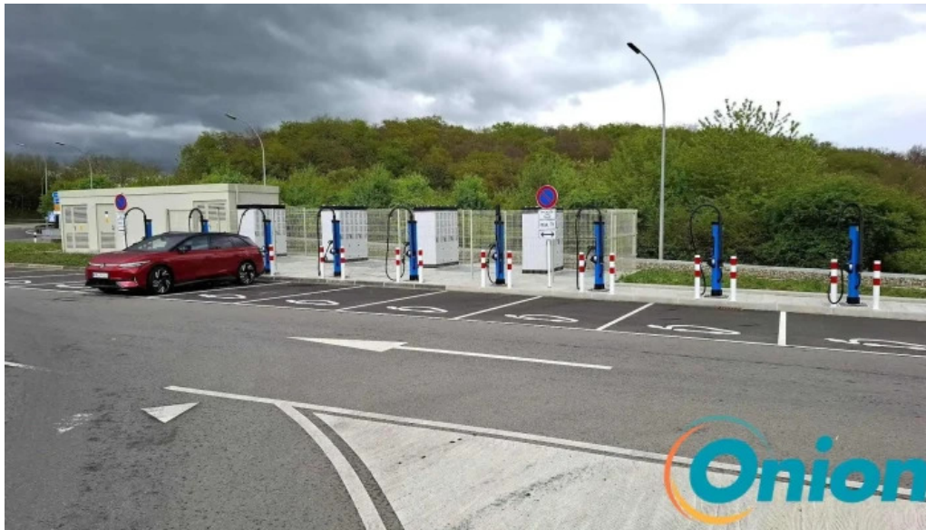
Chargy ladestation neueste
