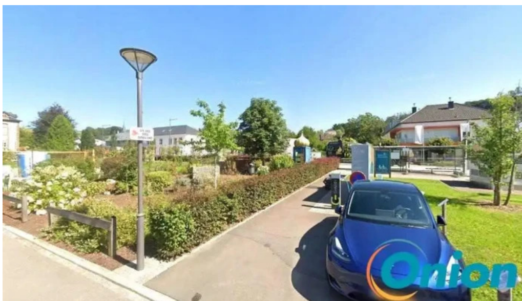
Chargy charging station preizerdau
