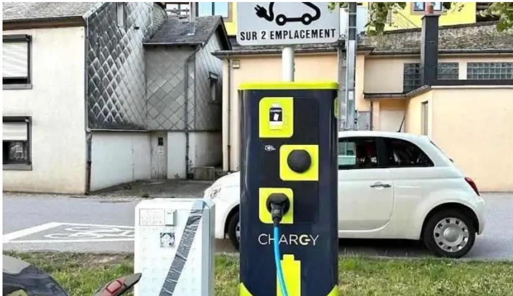
Chargy charging station rambruch
