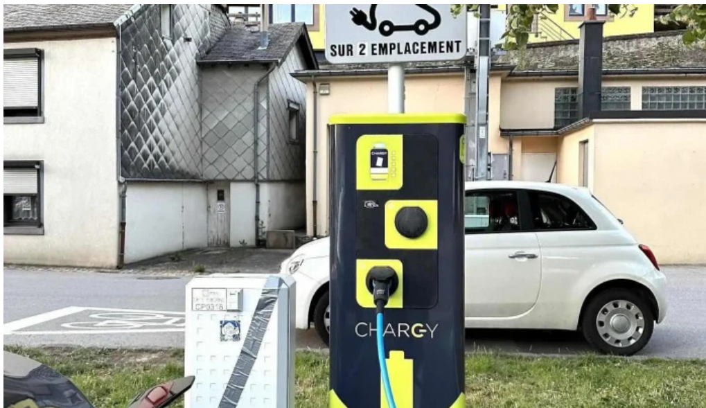
Chargy charging station praissere
