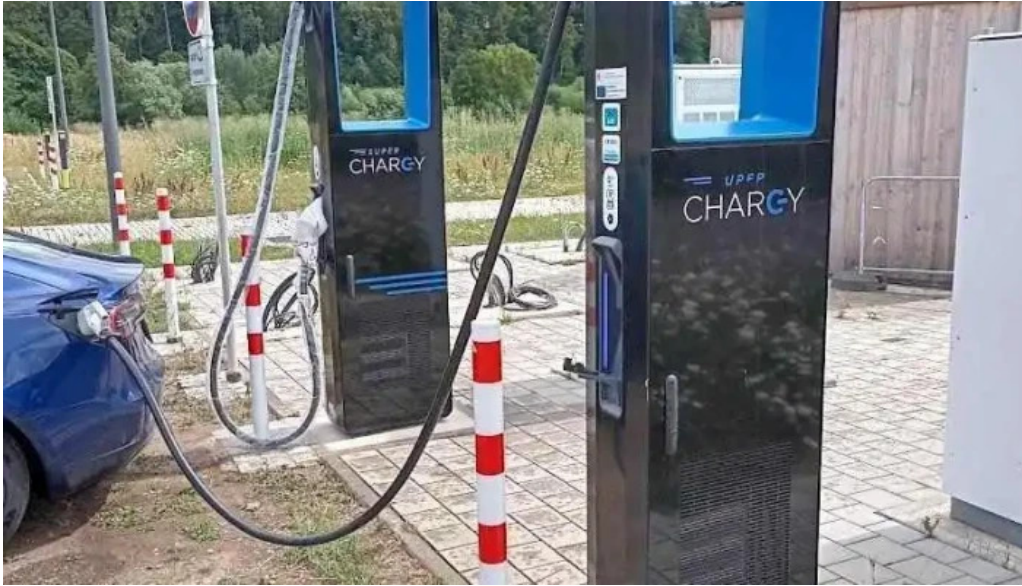
Charge charging station saeul
