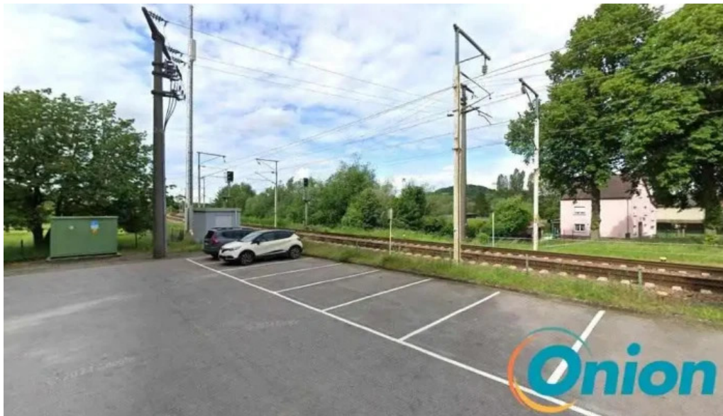
Chargy charging station schuttringen
