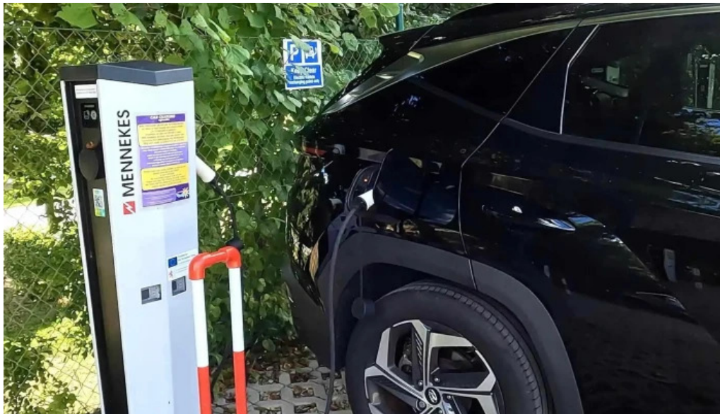
Chargy ladestation strassen
